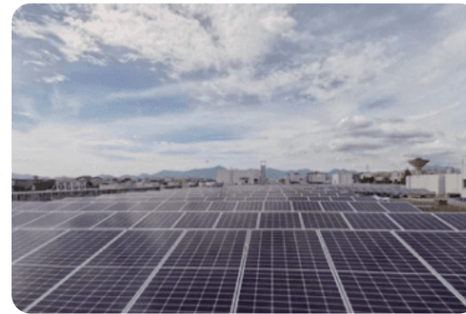
▲ Solar panels at CEM3
