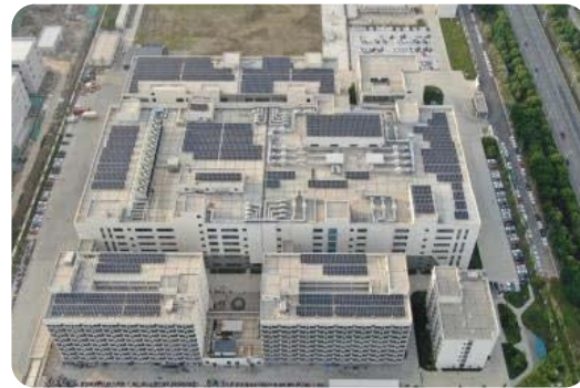
▲ Solar panels at CEM5
